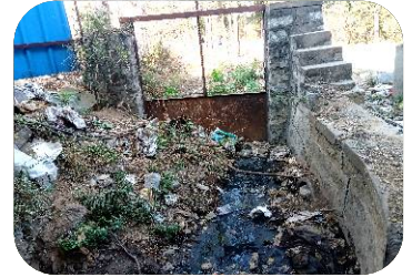
Broken/ dilapidated infrastructure
