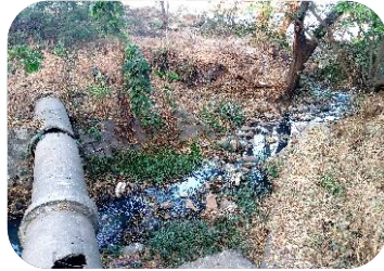
Broken sewage infrastructure adding to pollution
