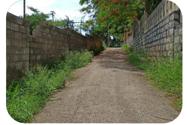
Encroachments on water paths
