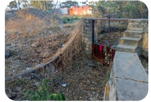
Broken infrastructure and lack of regular maintenance
