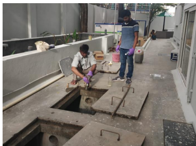
Water Sampling after Commissioning
